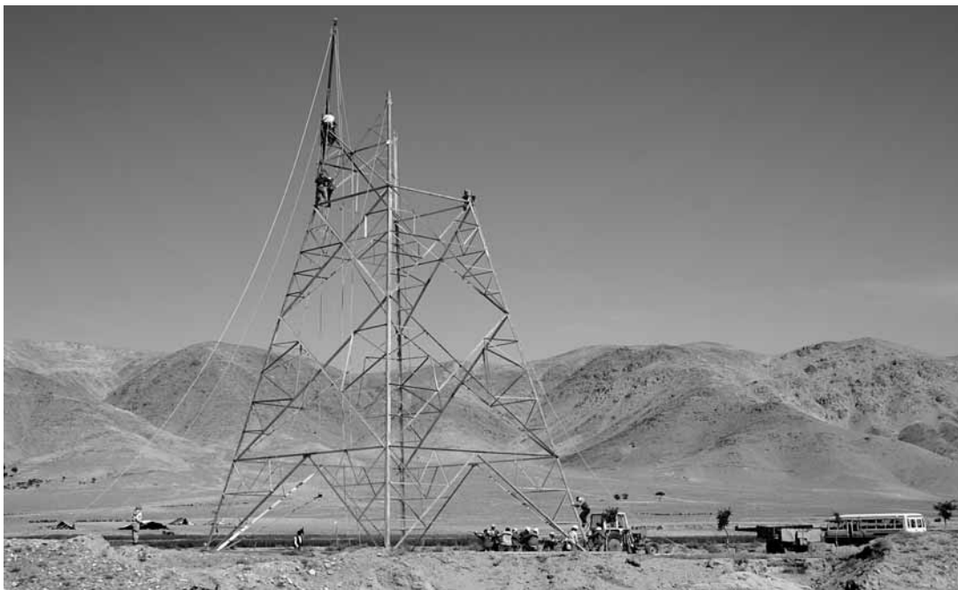
A group of the Indian electricity company electricians working on a electricity post along the Kabul-Parwan Highway.
